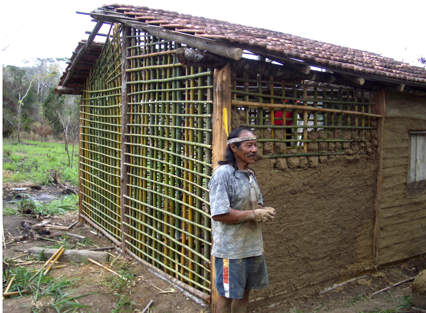
Figure 23.3: The former chief Jonas explains how to use raw materials (mud and bamboo) to build a more traditional Indian house, which has a lesser impact on nature. (Photo by Silva, 2008)
